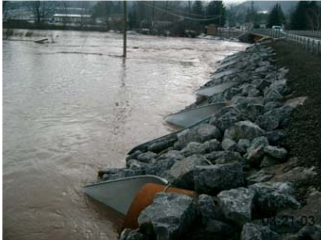
Figure 6.13 Floodplain relief culverts installed at County Bridge 2-1 in Delancey. Photo taken looking upstream, March 21, 2003
