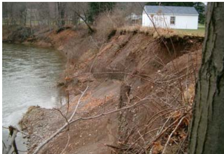
Figure 6.4 Severely eroding bank in the Village of Walton (December 2004).
