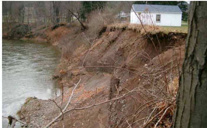
Figure 2.7 Closer view of the unstable embankment at the Terrace Avenue site (December, 2004).
