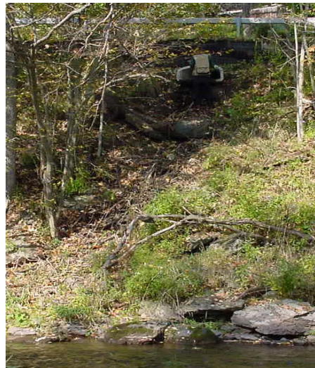
Figure 2.2 Poorly designed culvert outfall along NYS Route 10 upstream of Bloomville. Note direct discharge into river with lack of energy dissipation and sediment control measures. This site could benefit from a stormwater retrofit.
