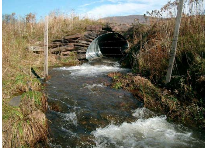
Figure 2.4 Culvert installation that could benefit from improved alignment, fish passage, outfall dissipation, headwall installation and top cover.
